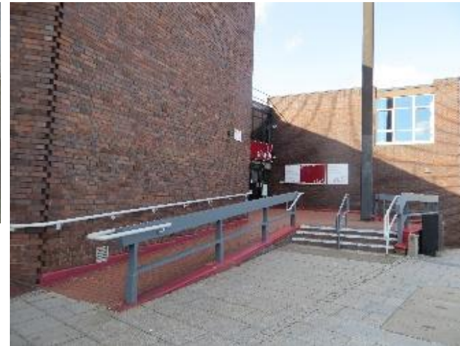
Slope or steps to access the front door on Moor Street Queensway
